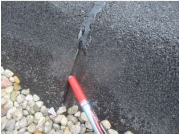
Photo #7 Typical view of perimeter flashing membrane starting to open
