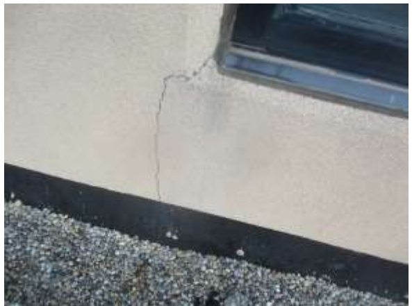
Photo #10 View of a typical crack below a window corner at the EIFS Gymnasium Wall.
