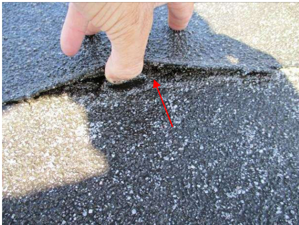
Photo #9 View of open modified membrane seam
