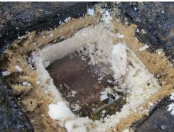
Photo #21 View of core cut with rusted deck and moisture in wood fiber board
