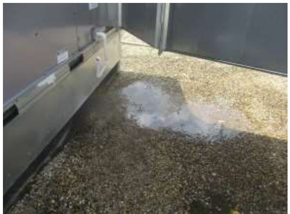
Photo #12 Typical ponding water near roof top units
