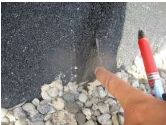
Photo #11 View of flashing membrane starting to open at gymnasium wall
