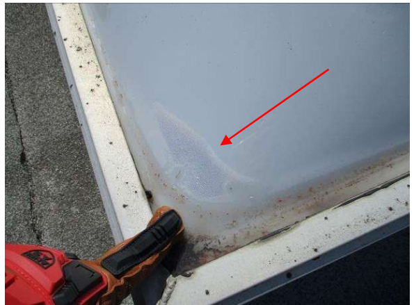
Photo #10 View of moisture on the interior of the skylight
