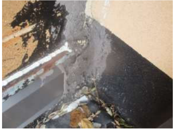
Photo #20 Typical view of previous roof cement repairs starting to open
