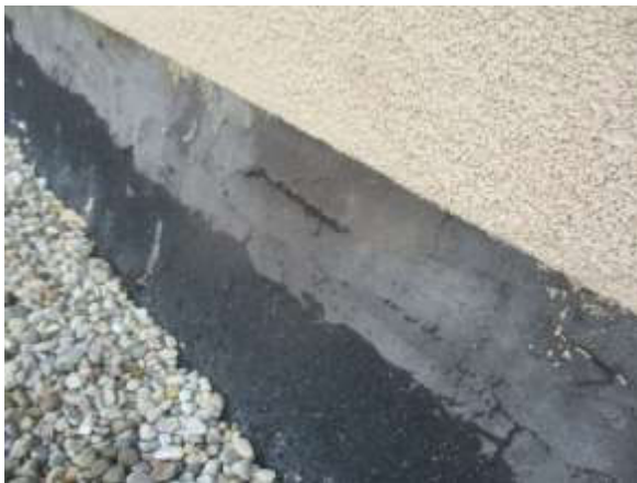
Photo #9 View of previous cement repairs at roof to gymnasium wall transition starting to crack and open
