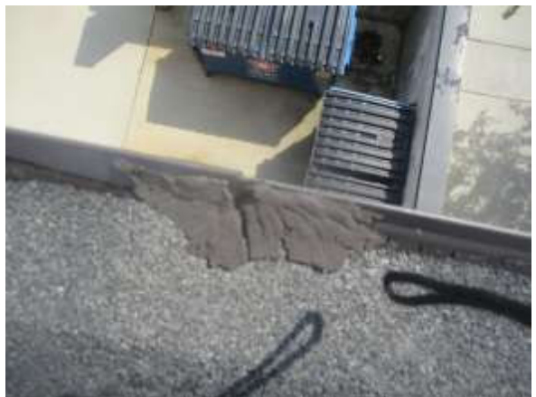
Photo #6 Typical view of previous cement repair starting to crack open
