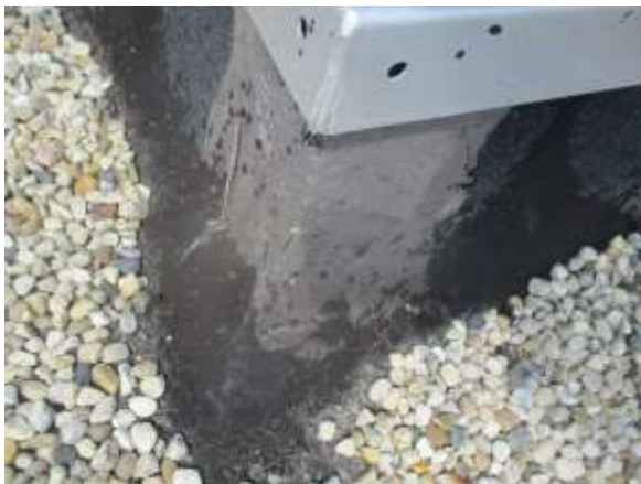
Photo #17 View of typical roof cement repairs at curb locations. Starting to crack.
