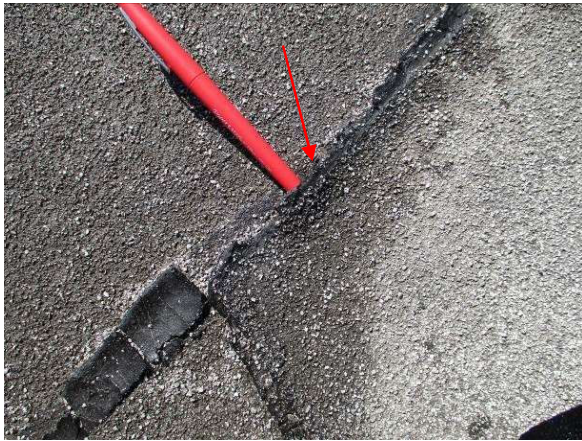
Photo #7 View of open modified membrane seam
