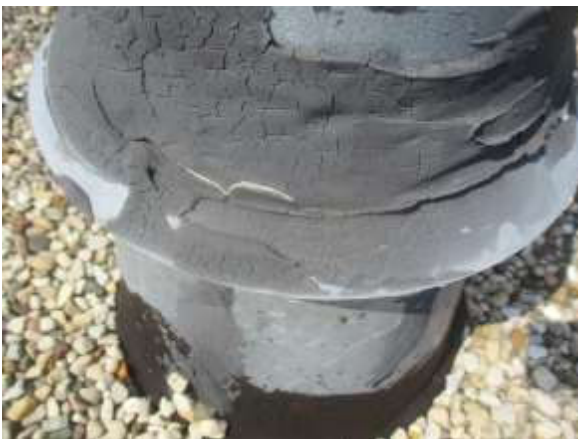
Photo #5 Typical view of weathered sealant at pipe penetration
