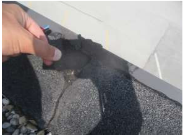
Photo #8 View of peeling perimeter flashing membrane
