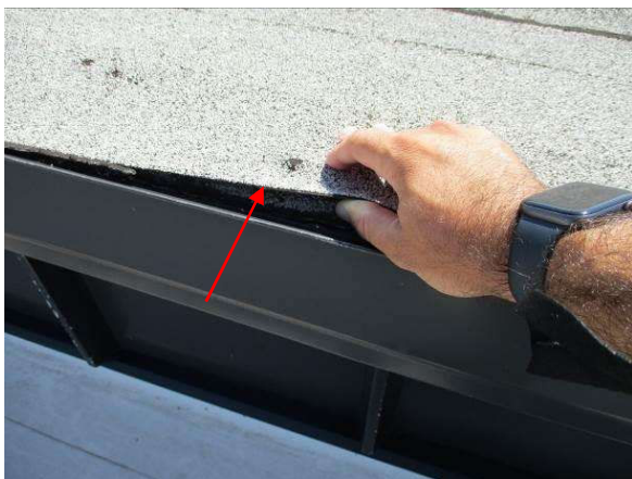
Photo #11 View of modified flashing ply at gravel stop not fully adhered
